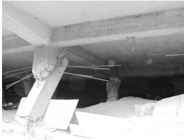
Figure 7. Buildings in Port Blair that were subjected to similar ground shaking intensity performed differently: a three-story RC-frame building collapsed in a brittle manner (photo: S. Jain).
