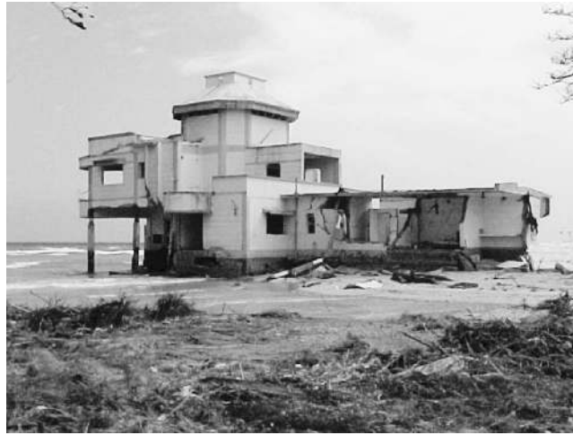
Figure 29. This RC-frame MES inspection bungalow now stands in waters at the Air Force Colony south of Malacca on the east coast of Car Nicobar Island (photo: C. Murty).
