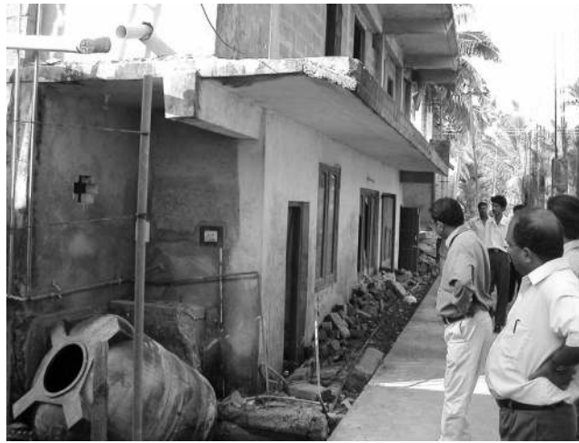
Figure 5. Settlement of RC buildings at Bamboo Flat near Port Blair (photo: H. Kaushik).
