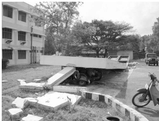
Figure 19. Collapse of a 2-m-high shelter for bicycles and motor scooters near the Port Management Board office complex in Port Blair (photo: S. Jain).
