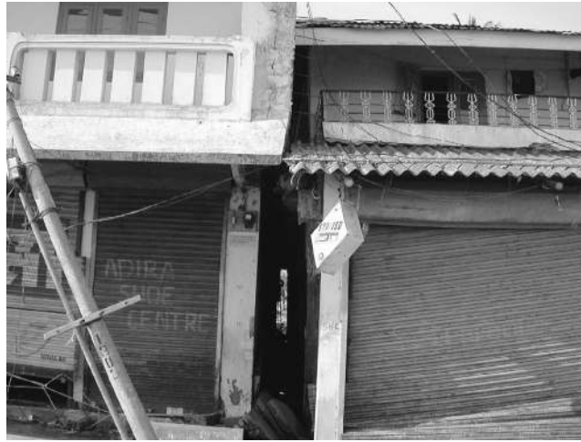
Figure 21. Pounding occurred between closely constructed buildings in and around Port Blair. These buildings are in the Bamboo Flat shopping complex (photo: S. Jain).
