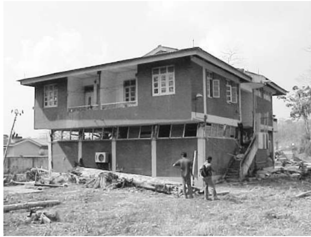
Figure 18. The BSNL telephone exchange building on higher ground at Hut Bay in Little Andaman Island was severely damaged due to earthquake shaking—it was twisted about the vertical axis during the shaking and sustained severe irreparable damage in its structural members. The structure was also flooded by the tsunami runup, and severe loss was sustained in non-structural elements and contents (photo: C. Murty).
