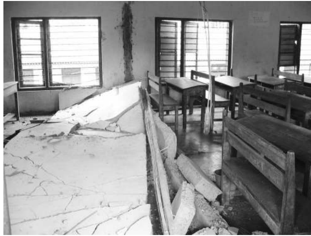
Figure 12. Slender masonry walls became dislodged because of out-of-plane instability and poor connection or no connection to the surrounding structural elements at the senior secondary school building in Adazigin, Middle Andaman Island (photo: D. Rai).
