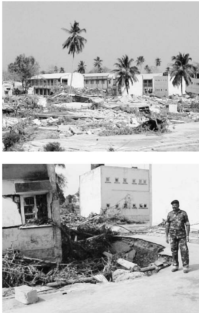
Figure 28. These buildings at the Air Force Colony in Car Nicobar Island are apparently standing after the tsunami, but their foundations have been scoured away (photos: C. Murty).
