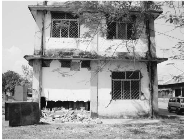
Figure 31. The old dry dock in the marine jetty dry dock complex was inundated in seawater after the event, and the masonry walls were damaged (photo: H. Kaushik).
