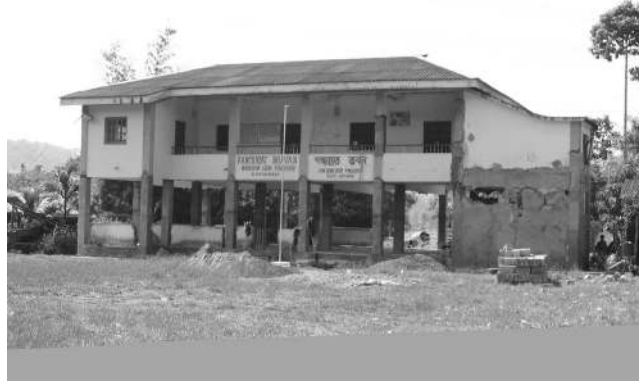
Figure 16. The Nabagram panchayat bhavan building was shaken by two earthquakes—on 14 September 2002 and 26 December 2004. Severe cracking and damage were observed in the soft first-story columns, and columns in the first story that were primarily damaged in the 2002 earthquake because of “missing” ties were now more severely damaged in the 2004 earthquake, even though they had apparently been “retrofitted” (photo: D. Rai).
