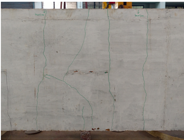
Fig. 8b Crack pattern seen in the panel F3.
