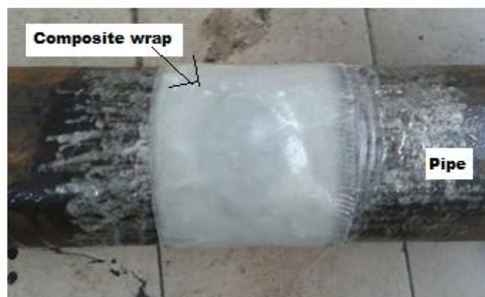
Figure 7. Circumferential slot defect repaired with elliptical configuration of metallic seal further reinforced with composite sleeve.
