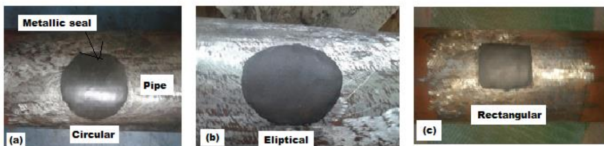
Figure 8. First phase repaired specimens of axial slot defect with different configurations (a) Circular (b) Elliptical (c) Round ended rectangle
