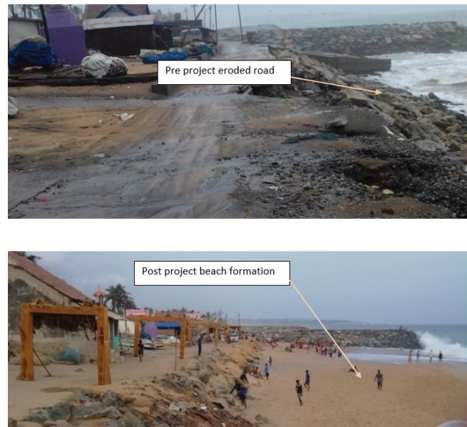
Figure 10. Beach formation along road which was eroded early
