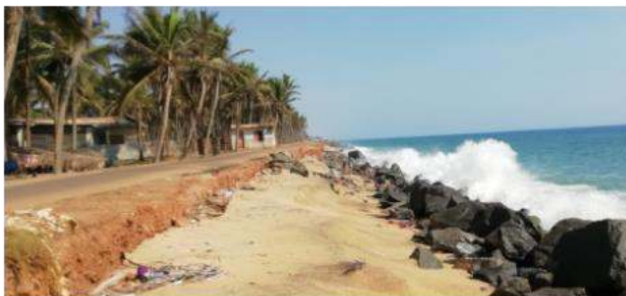
Figure 3. Erosion of coastal road
