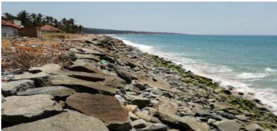
Figure 2. Sliding of existing seawall
